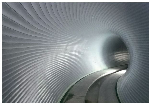
Jizomae rainwater trunk line for flood control
